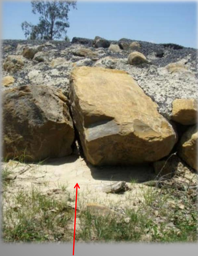
Loss of fines from scour
